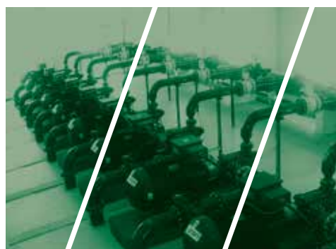
Boosting and Distribution of surface water
