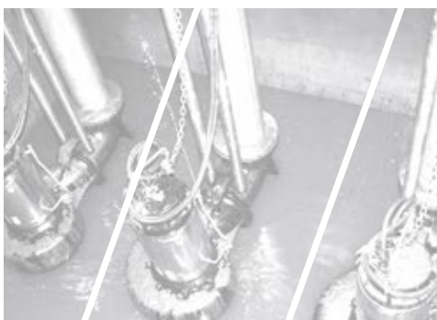
Wastewater Transport and Treatment
