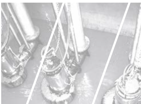
Wastewater Transport and Treatment
