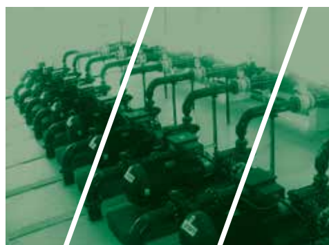
Boosting and Distribution of surface water
