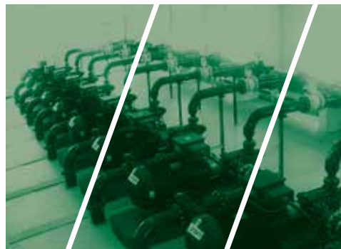
Boosting and Distribution of surface water
