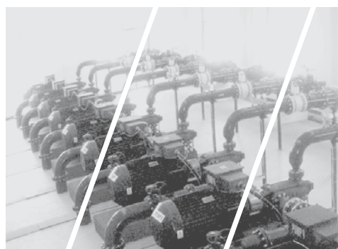
Boosting and Distribution of surface water
