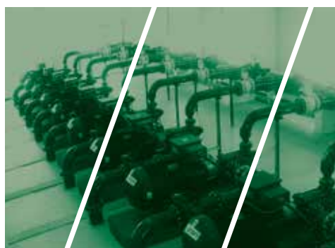
Boosting and Distribution of surface water
