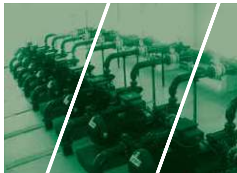
Boosting and Distribution of surface water
