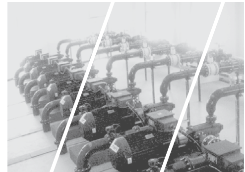
Boosting and Distribution of surface water
